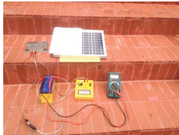
Fig. 9. Solar panel, DC Ammeter, Voltmeter, Battery, & Charge Controller used for data collection (with shading).
