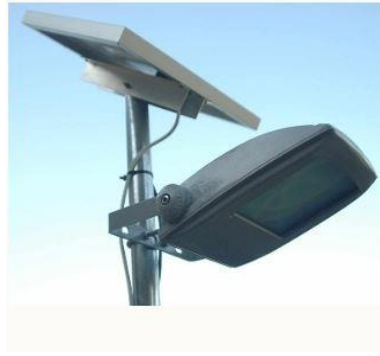
Figure 8 Solar floodlights with solar cell
