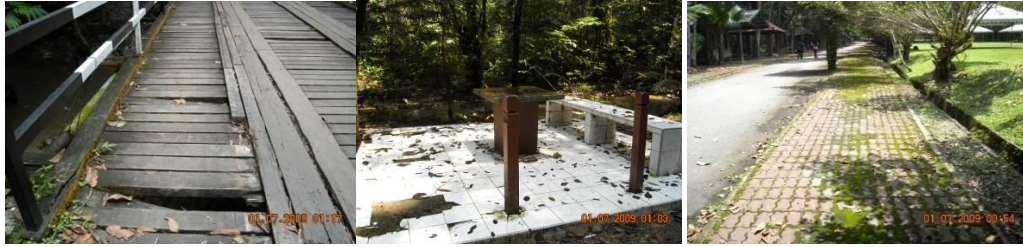
Figure 6: Some elements in Sungai Chongkak needs repairing and reconstruction works and wild grass on pedestrian walkway need to be clean off.
