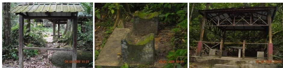
Figure 3: Poor maintenance causing damaged and unusable structures and equipment in Sungai Tekala Recreational Forest.
